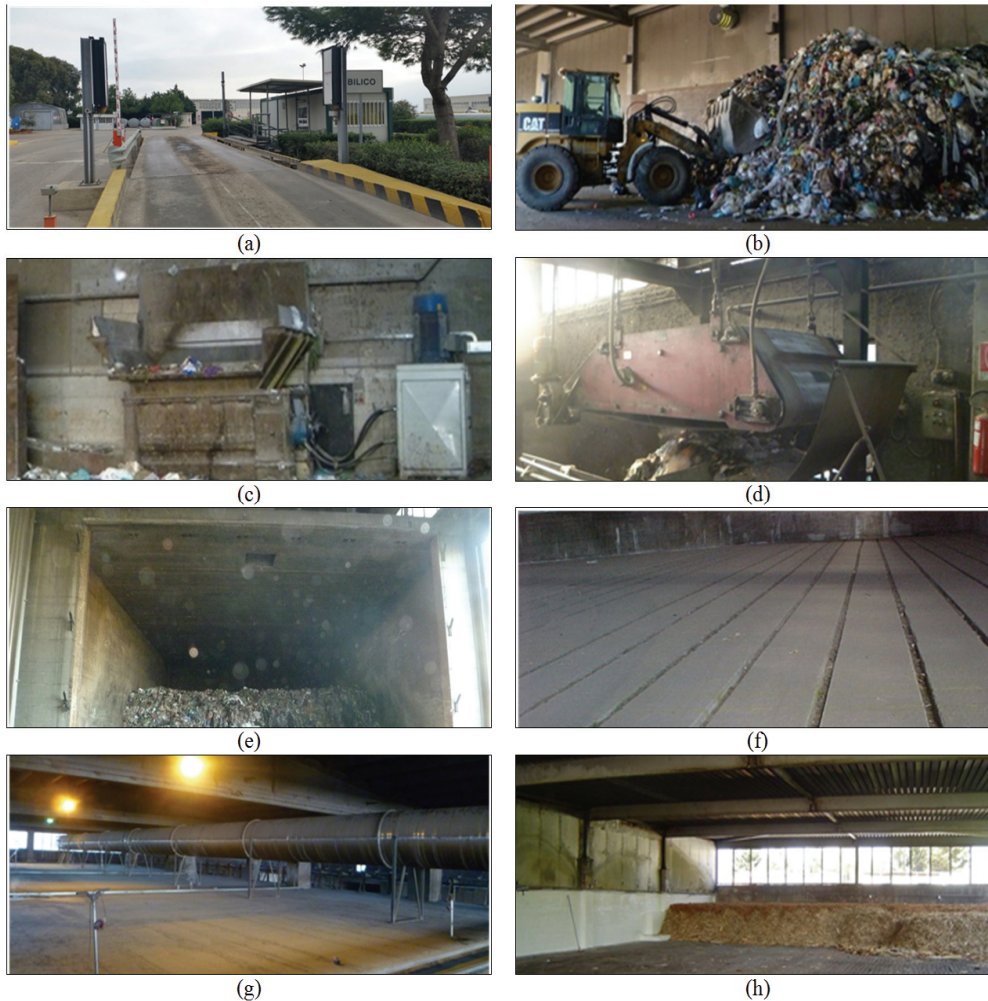
Fig. 1. CISA Spa MBT plant under investigation: (a) Acceptance and weighing of waste; (b) Waste storage in the reception area; (c) Primary shredder; (d) Iron separator; (e) Biocell; (f) Nozzles for blowing air on the floor; (g) Primary air pipe; (h) Biofilter
