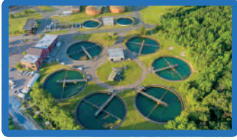
WATER MONITORING AND TREATMENT
